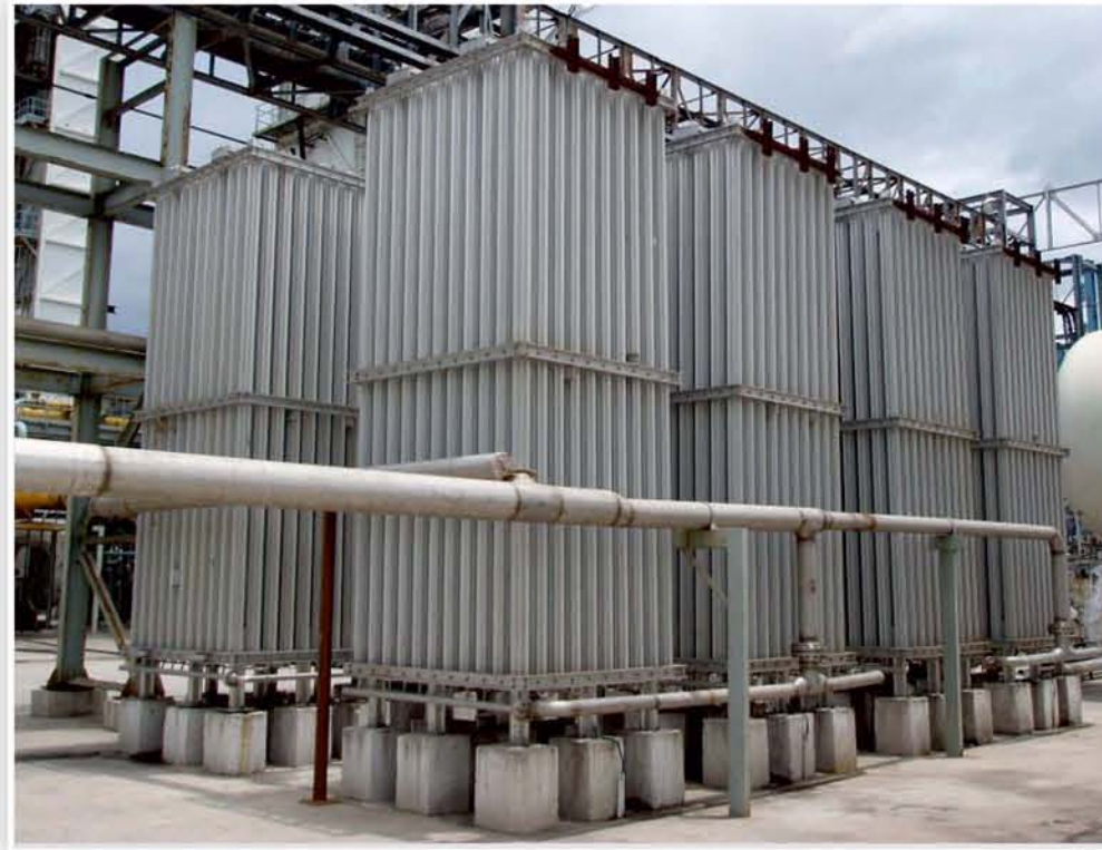
22000 nm 3 /hr . 30 bar, lox vaporizer for Steel Plant.
